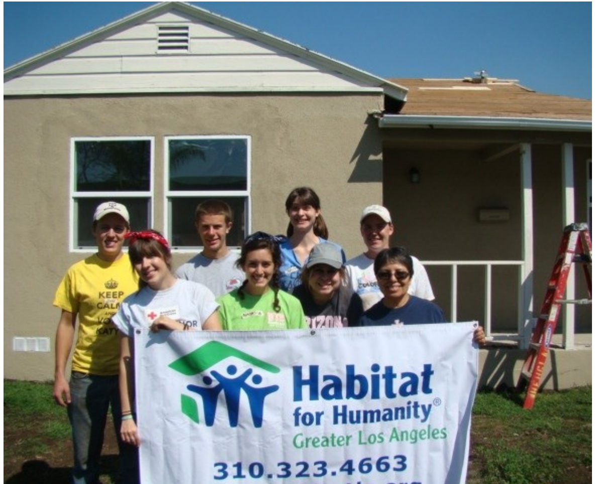
Sr. Angelica and 7 Newman students spent Spring Break working with Habitat for Humanity of greater Los Angeles. They worked on the roof of the depicted house near Long Beach.
